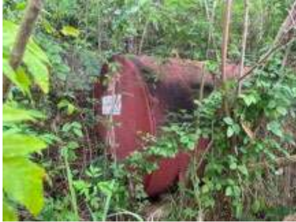
Existing 5,000-gallon fuel tank. No secondary containment, unknown if double-walled. Suspected to contain diesel fuel of unknown quantity.
