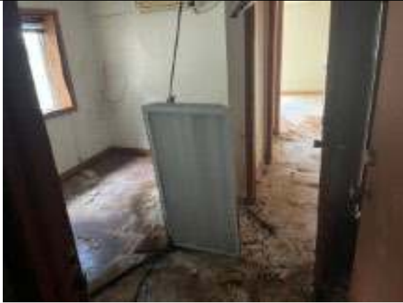
Suspected ACM material (floor tile). Suspected PCB ballast in light fixture.
