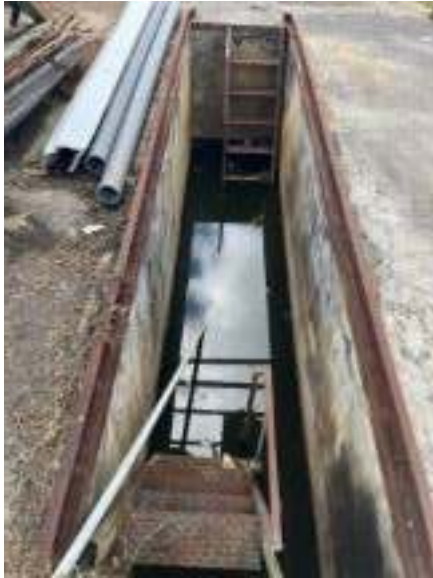
Vehicle Maintenance Pit with collected stormwater. No sheen or odor present to suspect contamination of water.
