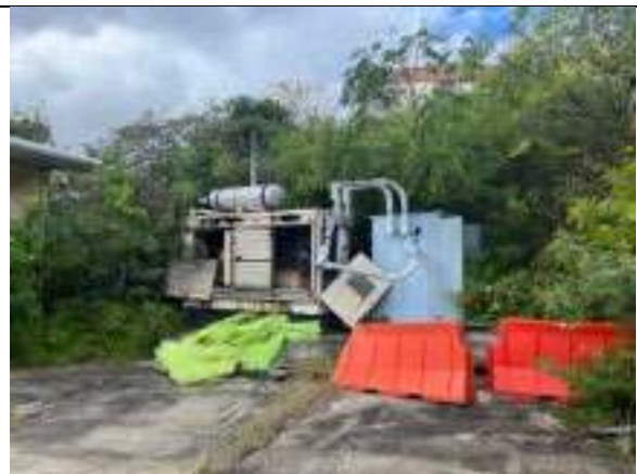
Existing emergency generator for site. Electrical switch gear suspected to contain transformer oil.
