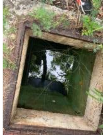
Sump/pit onsite with water. No sheen or odor present to suspect contamination of water.
